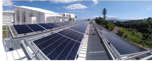
Figure 1 Installation photo and layout scheme. T indicates temperature probe, image of reference cell front-facing and rear-facing indicate their location. Each PV module is connected to an optimizer
